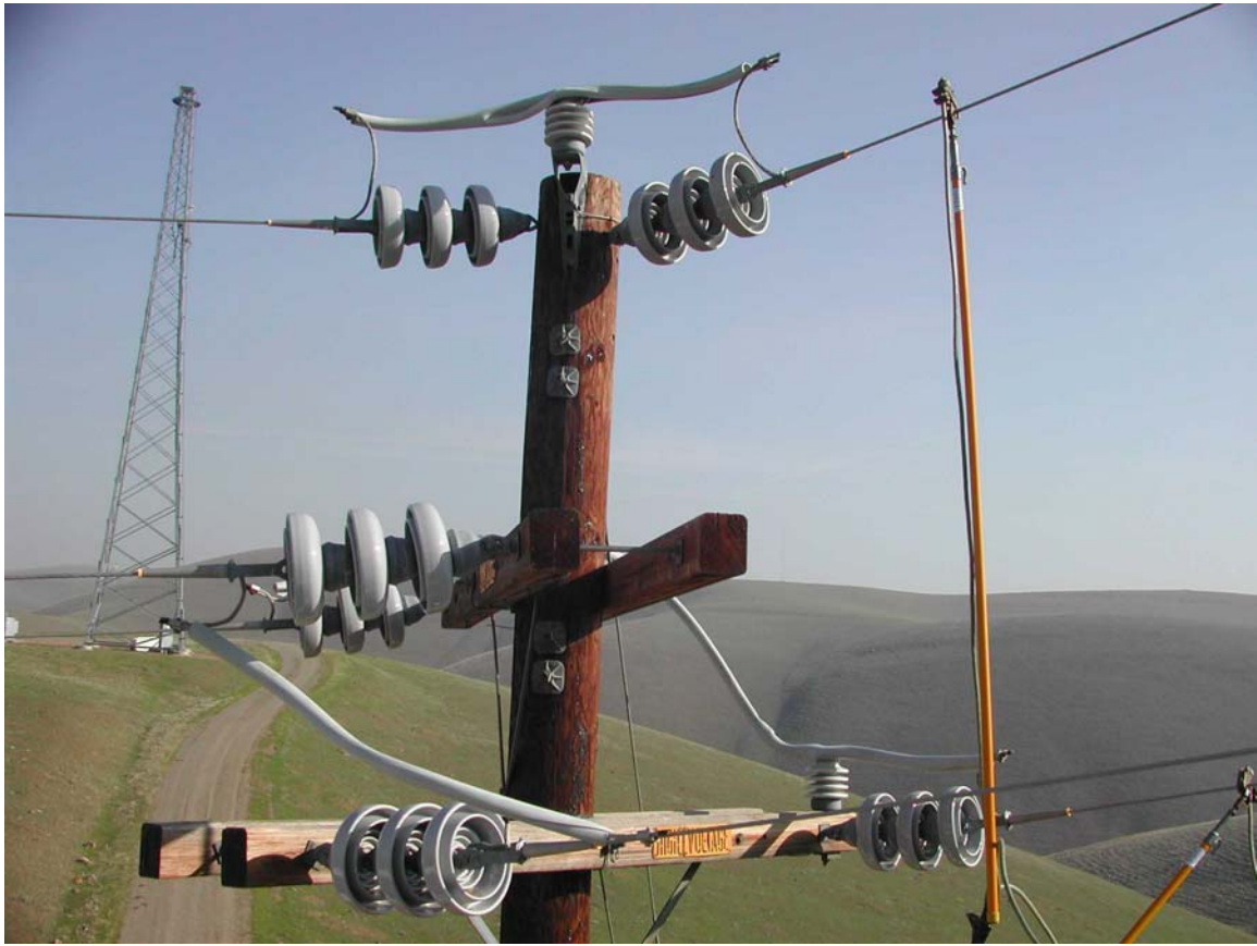
Figure 4. Typical corner pole with insulated wires.
