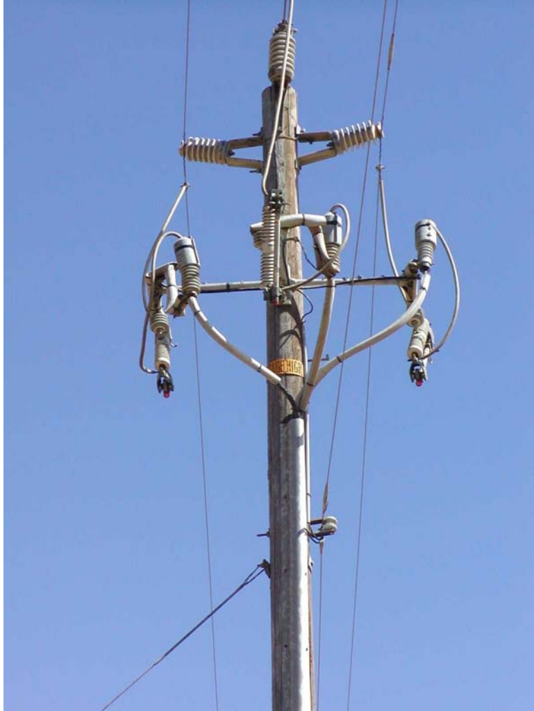
Figure 3. Illustration of a retro-fitted riser pole.
